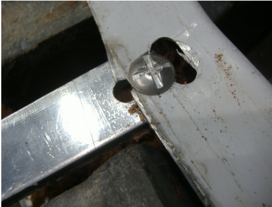
Plate 1 - Failure of Gutter at Bracket Connection
